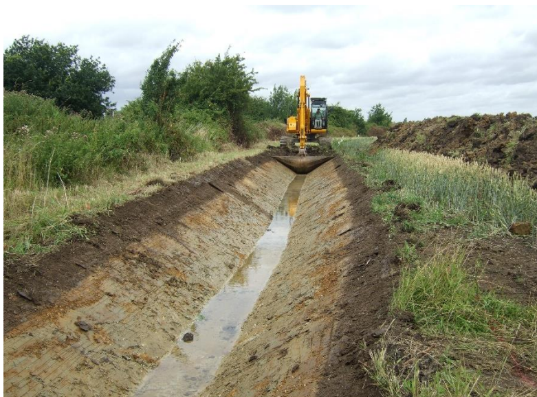
Figure 7-1: Completed action to create a new ditch near Eye Green to reduce flooding
